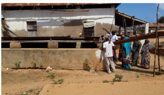
Dilapidated Djabia for rain water harvesting
