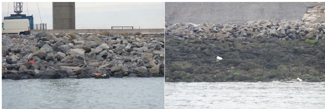
Figure 4: Plastic items between rocks of the harbour wall (inside) (Ostend)
