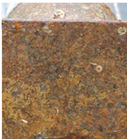
Fig. 5: Unprotected section of a UZ specimen after 36 months of exposure
