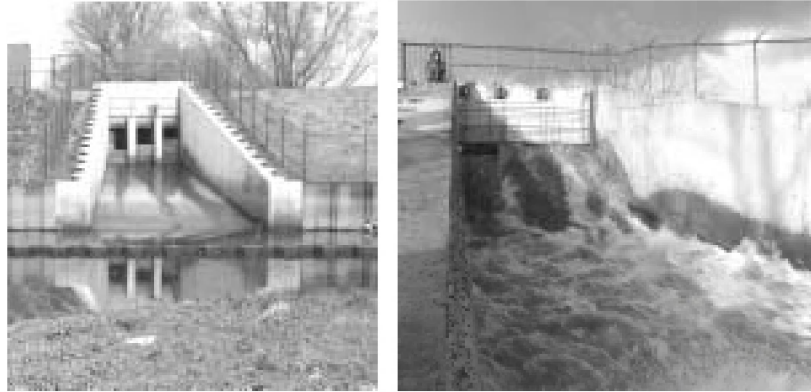
Photo 1.1 (left): Inlet culvert construction (as seen from within the pilot restoration site), consisting of three inlet culverts, each 1 m wide, with adjustable thresholds at different heights. Photo 1.2 (right): Close-up of the inlet culverts at spring tide flooding (as seen from within the pilot restoration site).
