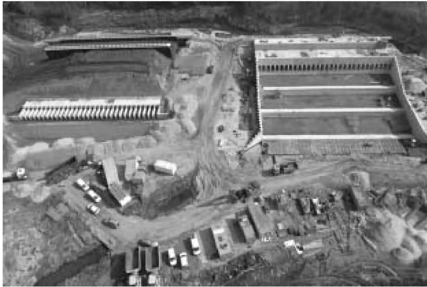
Photo 1.3: Aerial view of CRT construction along the Schelde. Photograph shows outlet (left) and inlet (right) construction which will allow implementation of CRT on several hundreds of hectares of lowered agricultural land.
