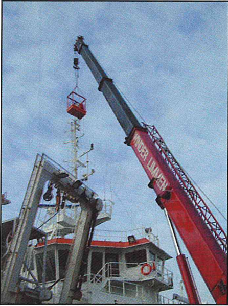
Changing a sensor is not an easy task when a sensor such as the anemometer is mounted on the top of a mast, 25 meters above sea level. (photo: Taco de Bruin)
