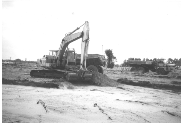
Fig. 3. 1999: The excavating of a fertilised area in D'Heye at Bredene to restore '2190 humid dune slacks' and '2150 EU-Atlantic decalcified fixed dunes ( Callunoa-Ulicetea )'.
