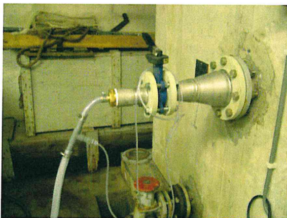
Figure 4 : Sampling point at tank 3
