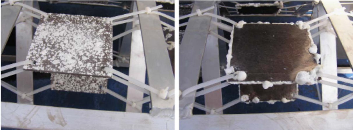
Figure 3.3-25 Examples of aluminium alloy specimens as retrieved from the sea after 12 months of exposure at a depth of about 3350 m within the KM3NeT framework. Left: Al 6082 T6 alloy showing typical pitting corrosion of aluminium alloys. Right: Al 6082 T6 hard anodized alloy, corrosion products affects only the margins where the surface treatment is weaker.
