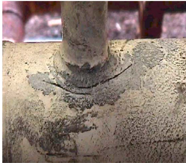
Figure 3-7 Corrosion fatigue sample[2].
