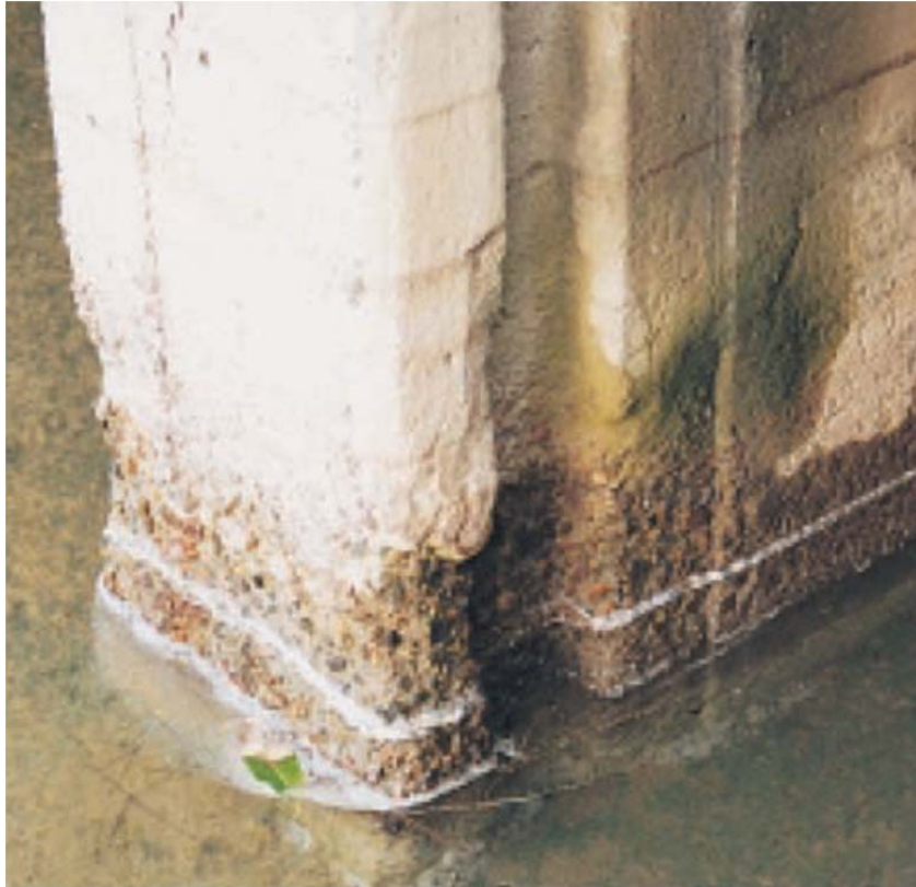
Figure 3-26 An example of where acid water derived from acid sulphate soils has corroded concrete.
