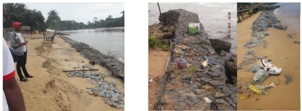
Figure 19. Construction of a protective dyke at the Lobé waterfalls in Kribi. (Credit: Mbevo, 2017; Tchindjang, 2013).
