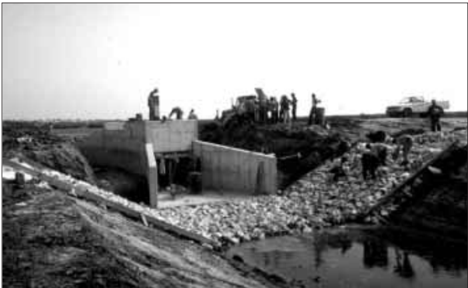
Picture 5: Construction of the Lekser sluice-gate. This was one of two sluice-gates added to the original scheme on the advice of the local fishermen.
