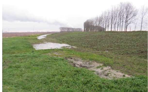
Figure 2 The new dike in the south of the Dutch Hedwige polder under construction. Photo by K. van den Hoven.
