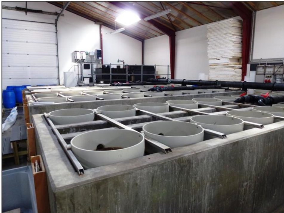
Figure 33: The concrete troughs containing microalgae-enriched production water. Inside hang the sieve-like round containers with the spat.
