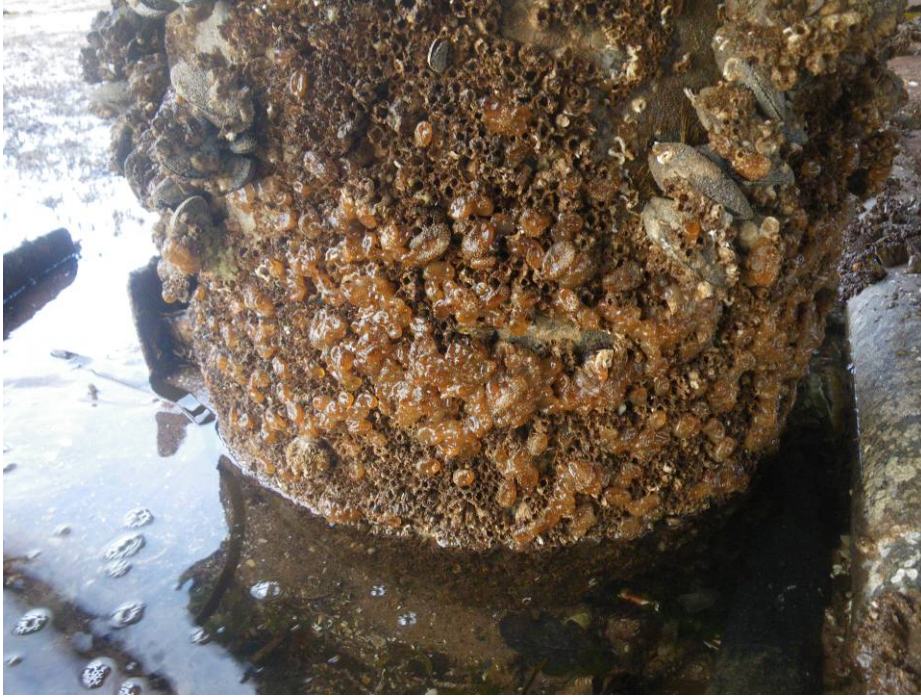
Photo 3.13 Corella eumyota at the base of a piling under Wemyss Bay Cal Mac pier. (C. Beveridge, SAMS).
