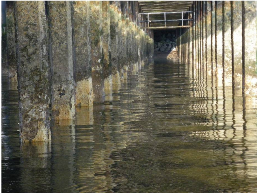
Photo 3.7 D. vexillum seen as creamy areas at the water line on the left hand pilings of Fairlie Quay Jetty (C. Beveridge, SAMS).
