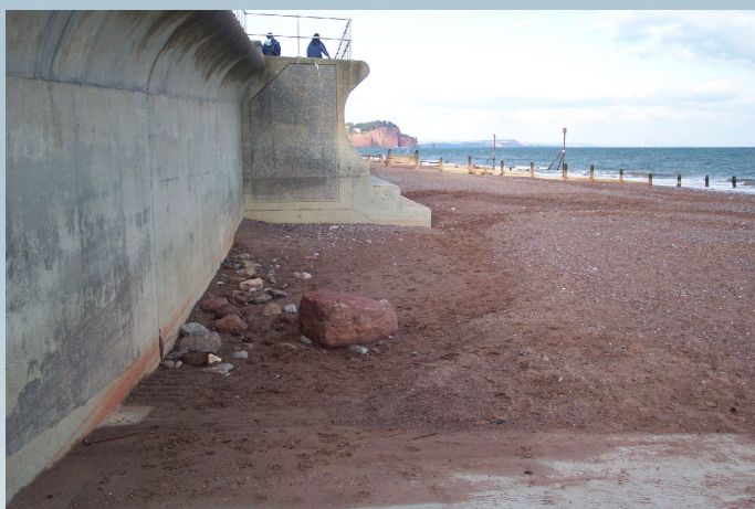
Fig 1. Seawall at Teignmouth, beach levels lowered in front of seawall affecting flood risk (courtesy of Dominic Reeve, University of Plymouth)
