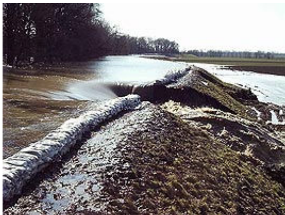
Fig. 2. Dike failure at Tarpa, Upper-Tisza, Hungary, March 2001 (photograph courtesy of Iván Kántor)
