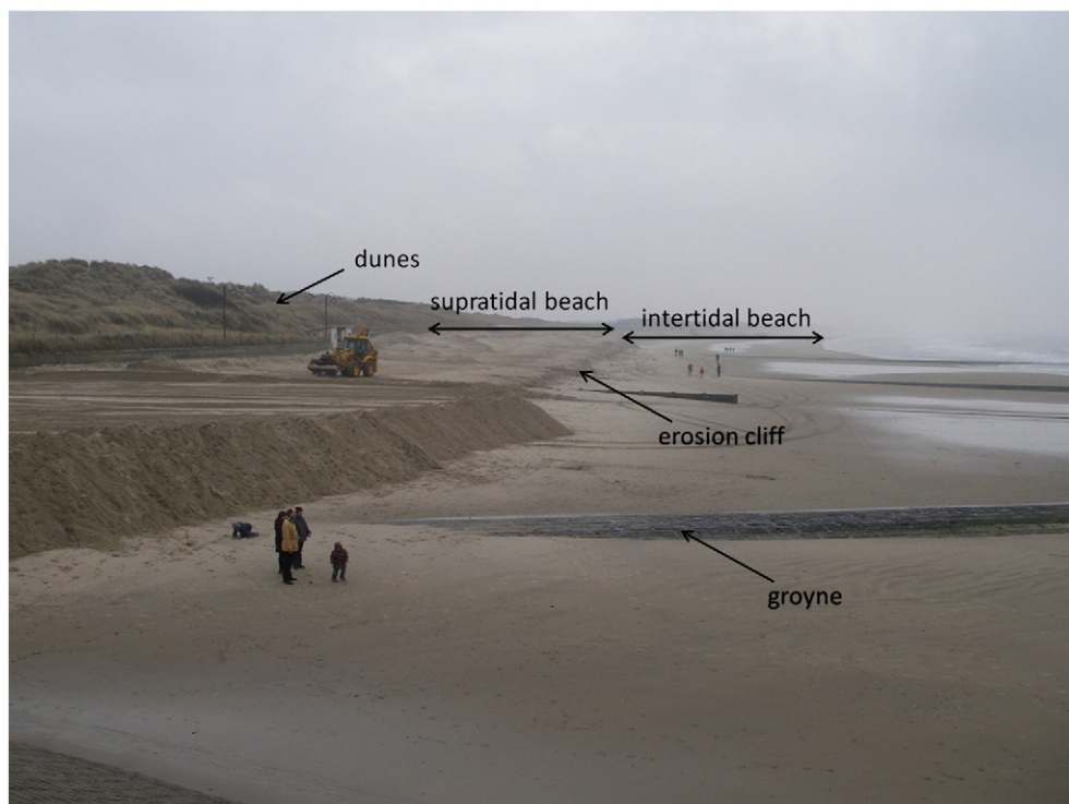
Fig. 13. Part of the beach west of Wenduine (March 2008) (photo by IMDC, 2008). The supratidal berm is rebuilt artificially each spring, after the winter storms.
