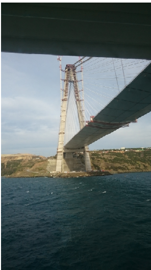
The bridge under construction at the Black Sea end of the Bosphorus
