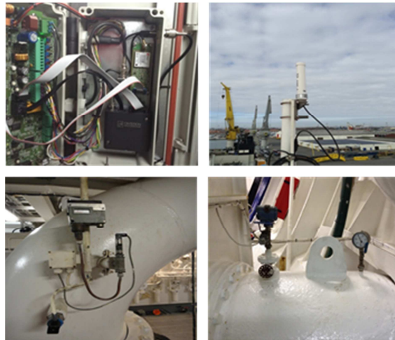
Figure 3: An installed EMS 2.0 system and its sensors
