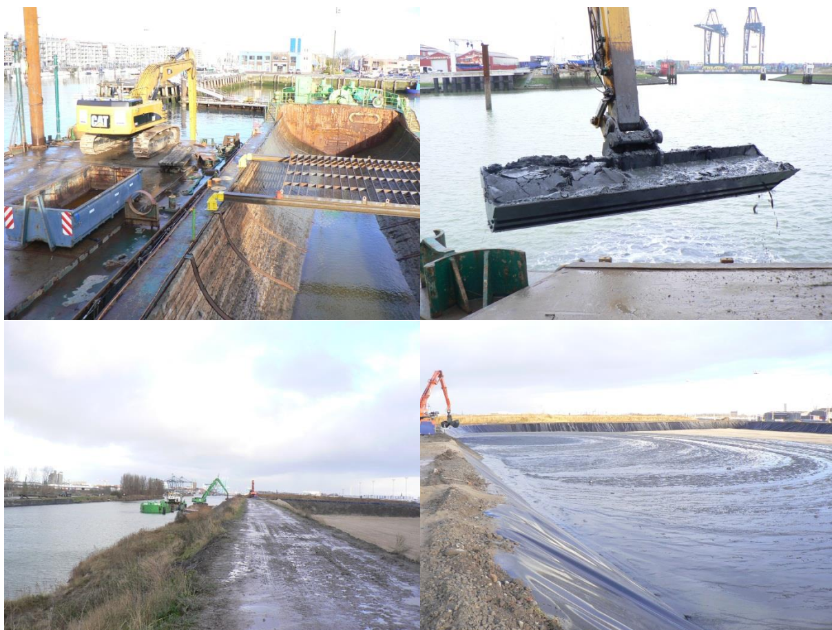
Figure 6.6: Dredging works of contaminated sediments in the Tidal dock of the old fishing harbour in Zeebrugge (upper) and the lagoon site for the polluted material in the inner port of Zeebrugge (below).
