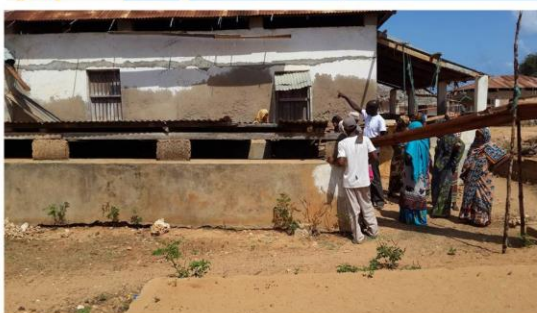
Dilapidated Djabia for rain water harvesting
