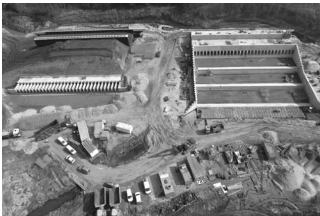
Figure 2: Aerial view of current CRT construction along the Schelde. Photograph shows outlet (left) and inlet (right) construction which will allow implementation of CRT on several hundreds of hectares of lowered agricultural land. Riverside dike is situated above in the photograph.
