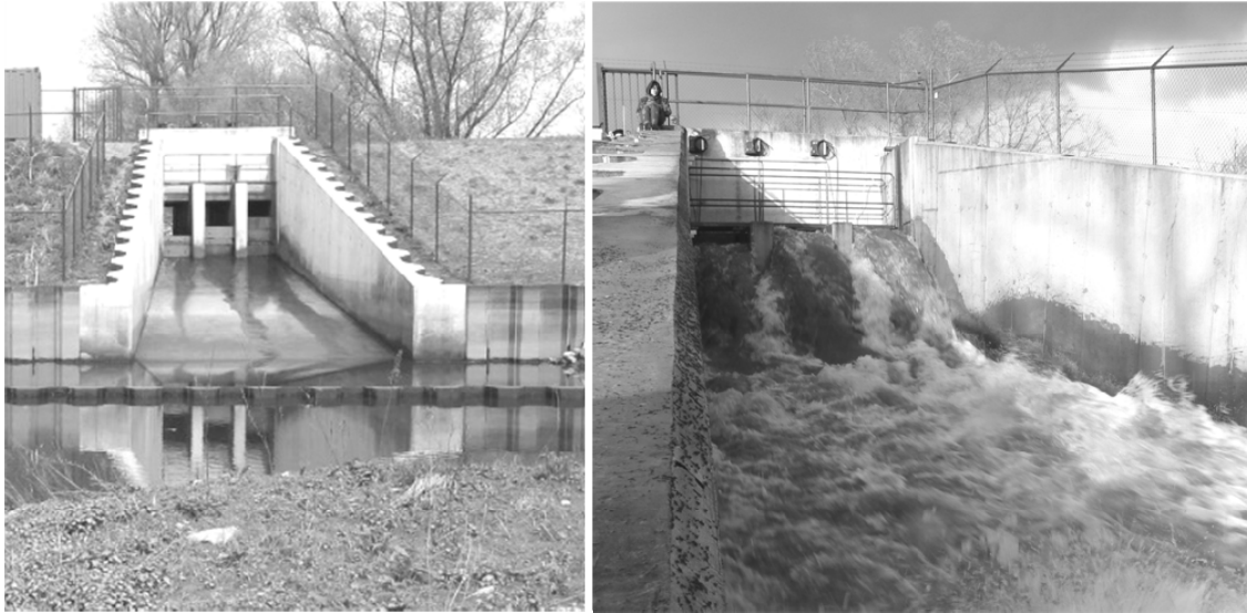
Figure 3 (left): Inlet culvert construction (as seen from within the pilot restoration site), consisting of three inlet culverts, each 1 m wide, with adjustable thresholds at different heights. Figure 3 (right): Close-up of the inlet culverts at spring tide flooding (as seen from within the pilot restoration site).
